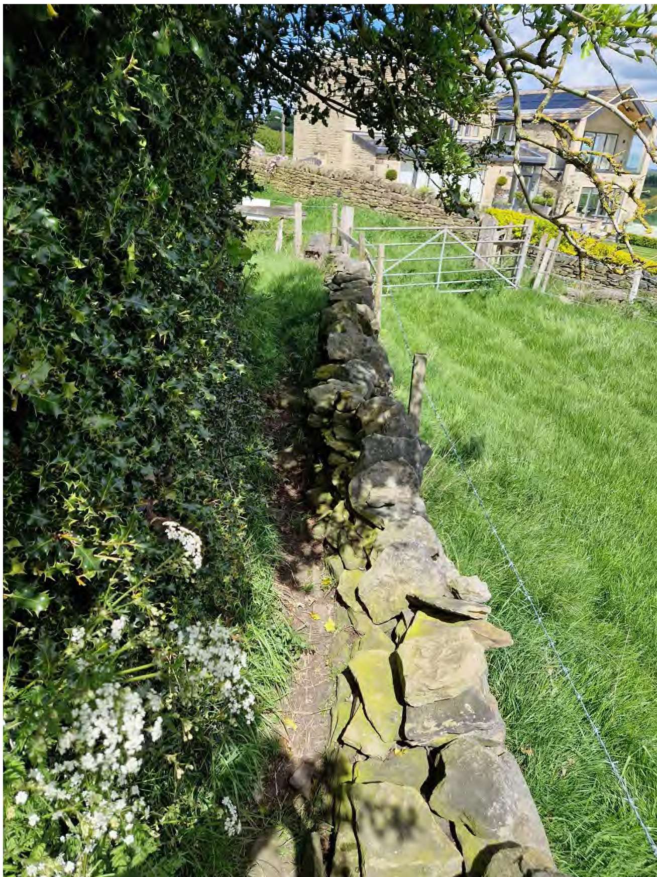
Photo 20: The width of the Order is severely limited by overgrown hedge near its junction with Crab Lane.
